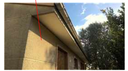
Façade Sud Plaques amiante ciment
